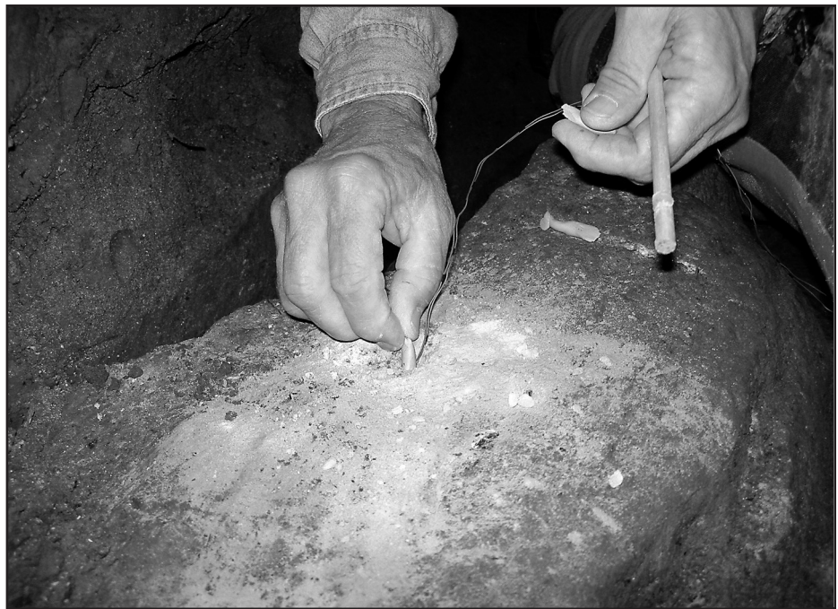
Figure 1. Rock shaving techniques using soda straws filled with pistol powder and inserted into a drilled hole in the rock create a very controlled splitting or shaving of the rock without the potential damage associated with more traditional explosives. Photo by W.K. Jones
