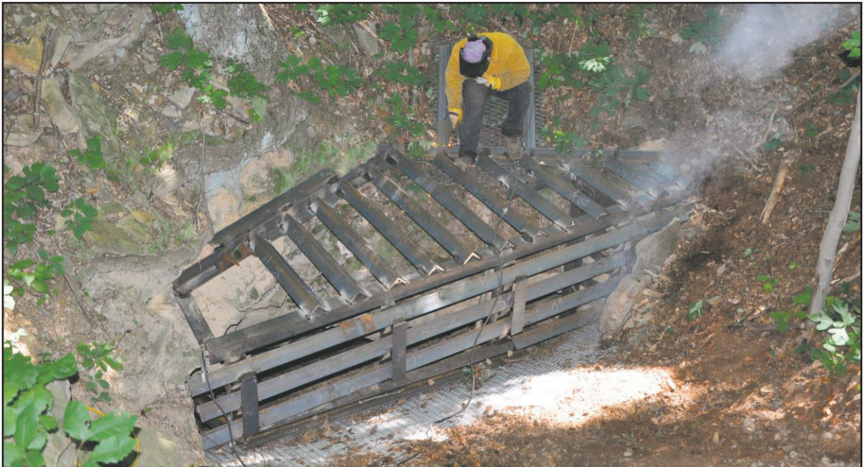
Folded Gate (in progress) on Dunbar Corporation Mine #3, Pennsylvania. Photo by Jim Kennedy.
