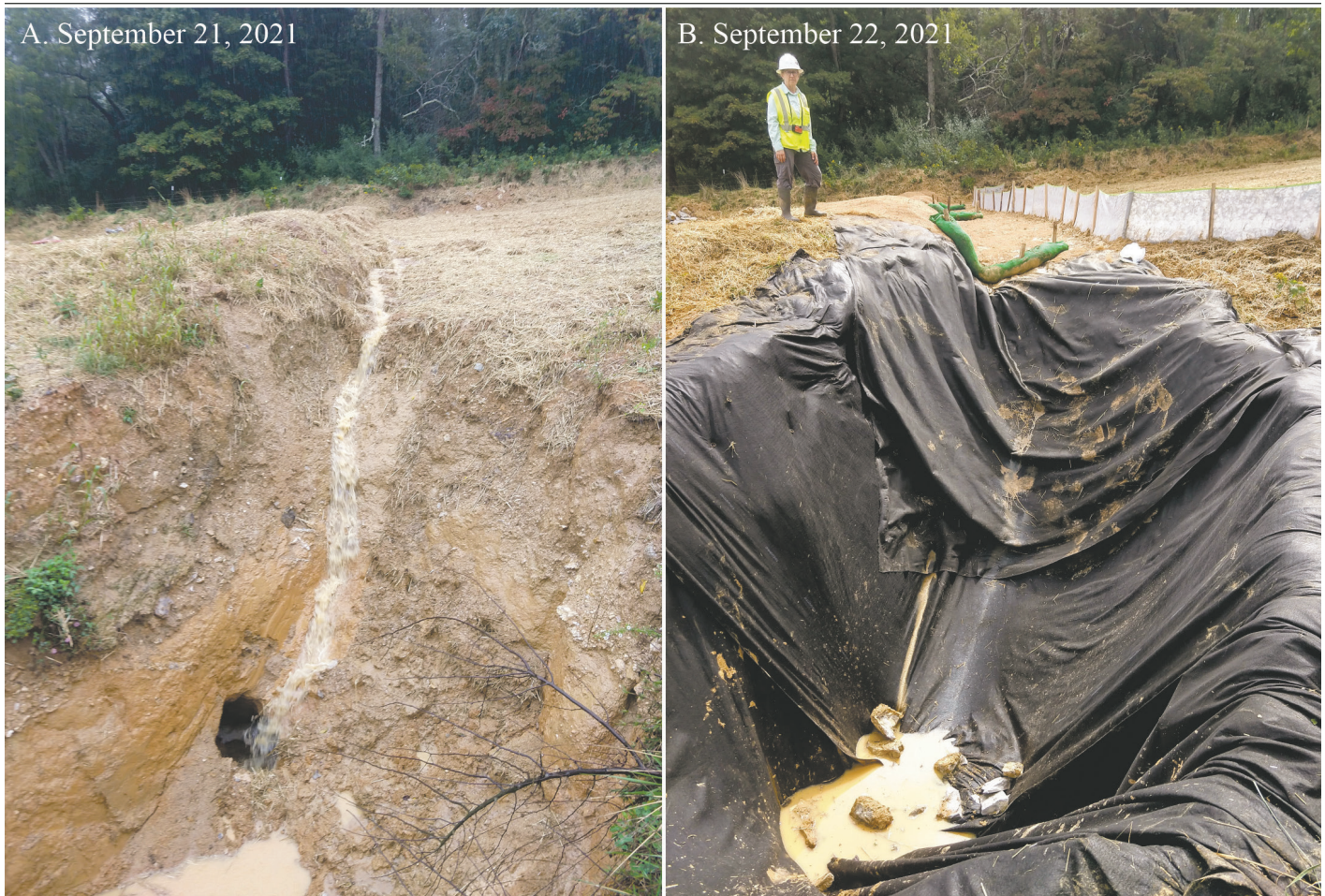
Figure 9. Intermittent swallet (A) and temporary stabilization (B), of the collapsed sump at the end of water bar, Mountain Valley Pipeline, Giles County, VA.
