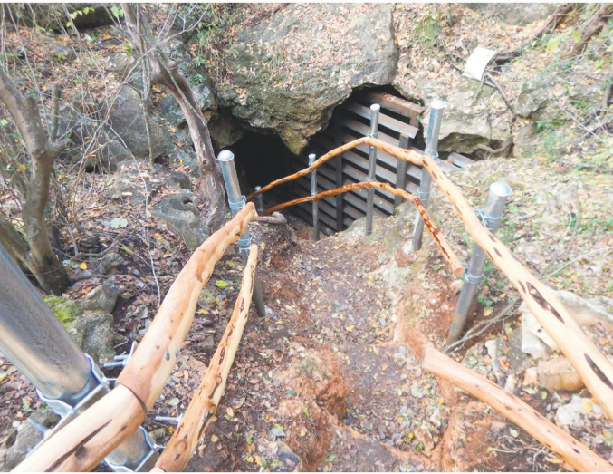
Figure 25. Installed gate, steps and guardrails at La Crosse Cave. Photo by Nico Hauwert.
