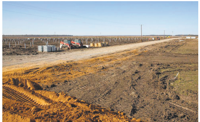
Figure 1. Solar sites during construction present the greatest risk to the site development and the karst resource, especially if sediment and erosion control is not properly planned and managed.
