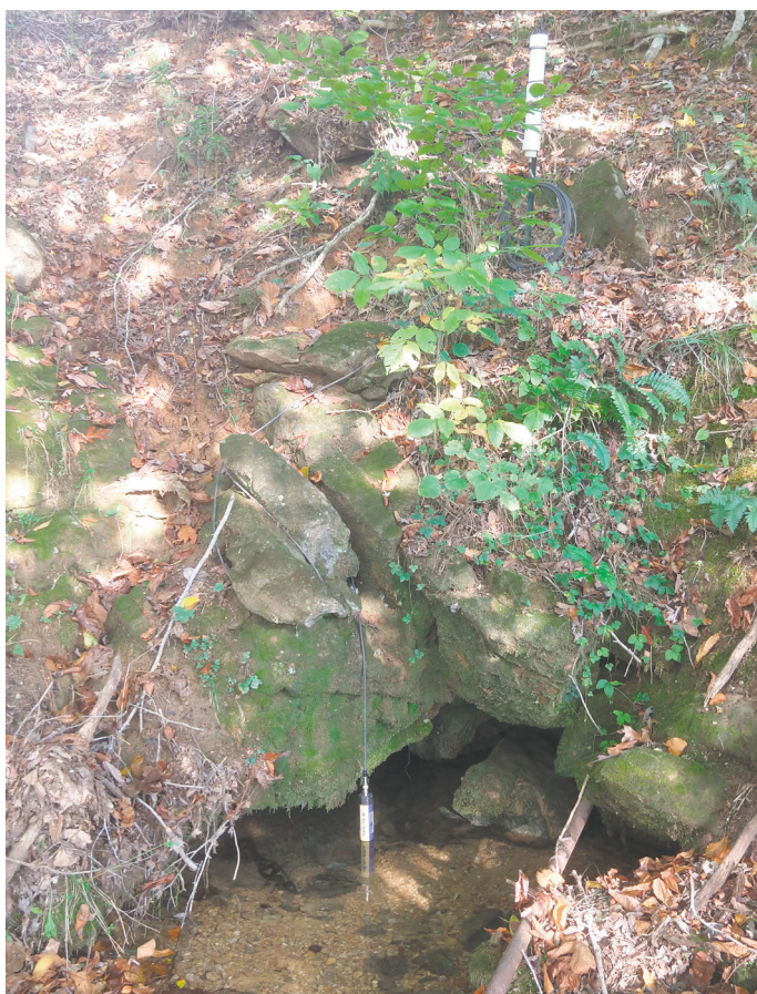
Figure 4. Water quality monitoring and telemetry installation, Canoe Spring, Giles County, VA.
