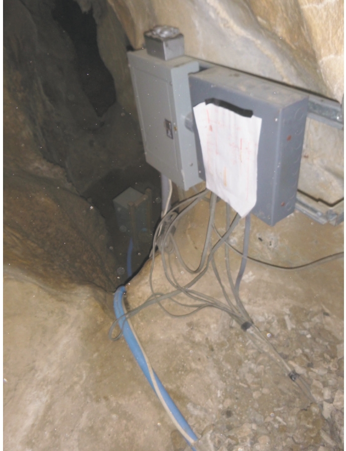
Figure 3. Electrical relay panel in the Doghouse, Lehman Caves, site for the data logger recordings in this article.
