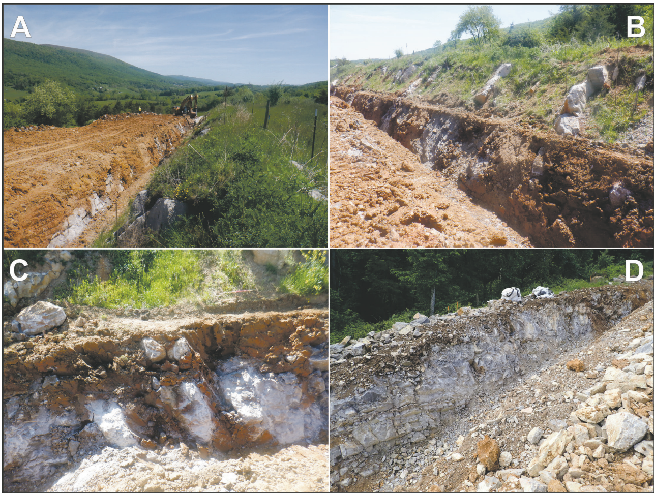
Figure 3. Exposed pipe trench (June, 2021) in area of 2019 sinkhole swarm along Mountain Valley Pipeline, Sinking Creek Mountain, Giles County, VA: A) overview of the trench in the area of the sinkhole swarm looking east, B) trench at the base of karst pinnacles exposed during grading, C) pinnacles with residual clay fill, D) limestone exposed in the trench along the slope just east of the area with the sinkholes.
