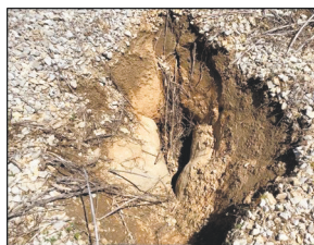
Soil/rock = 2 (failed backfill)
