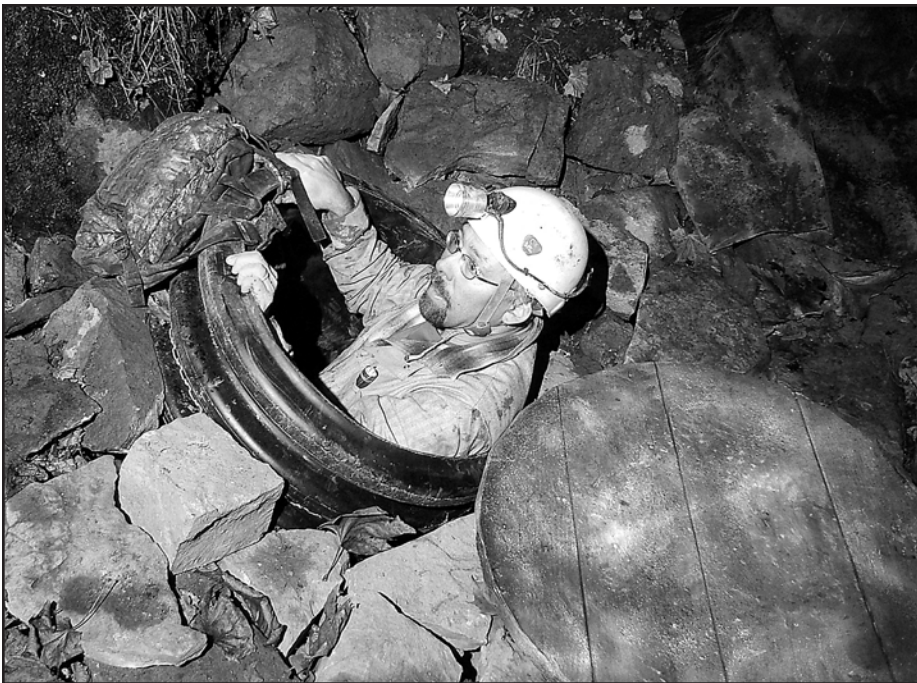
Figure 3. Dug entrances may be stabilized using culvert pipe. A lid may be fitted to control air flow and temperature fluctuations. In most cases, the management objective at the new entrance will be to maintain the cave in the same condition as before the new entrance was opened. In this example surface disturbance and visual impact are minimal. Photo by P.C. Lucas.
