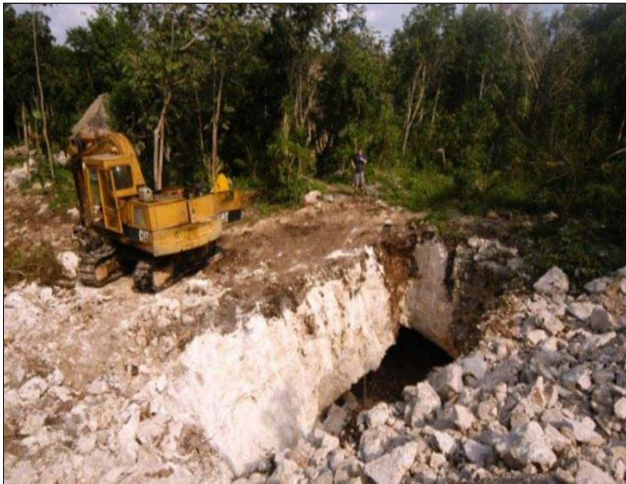
Figure 2 Recent example of cenote enlargement using heavy machinery. The landowner created an open water pool to attract paying snorkelers. (Photo by Robbie Schmittner)
