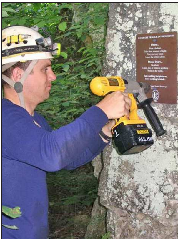
Figure 7 CRF worker installing a cave sign.
