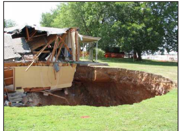
Figure 12 The collapse structure developed in a structured reddish-brown, cherty, and clayey residuum as can be seen from this view. From the angle of this picture the lack of subsidence of the area is apparent. Also visible is an abandoned steel septic tank.
