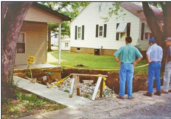
Figure 5A Collapse in residential neighborhood, Farmington, Missouri. This collapse had been repaired with soil fill only, but it reactivated.
