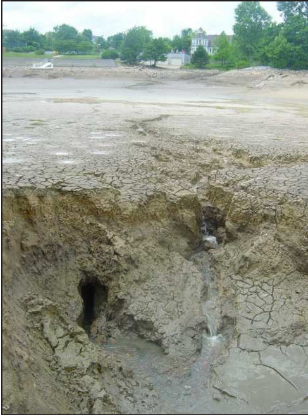
Figure 6C Soil cover collapsed beneath Lake Chesterfield into a well-developed cave.
